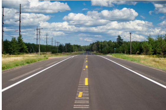
Figure 1. Center line rumble strip on two-lane roadway.
